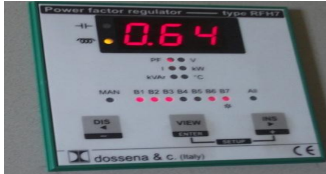
Figure 5.1: Capacitor stages C4, 5 are out of service.
